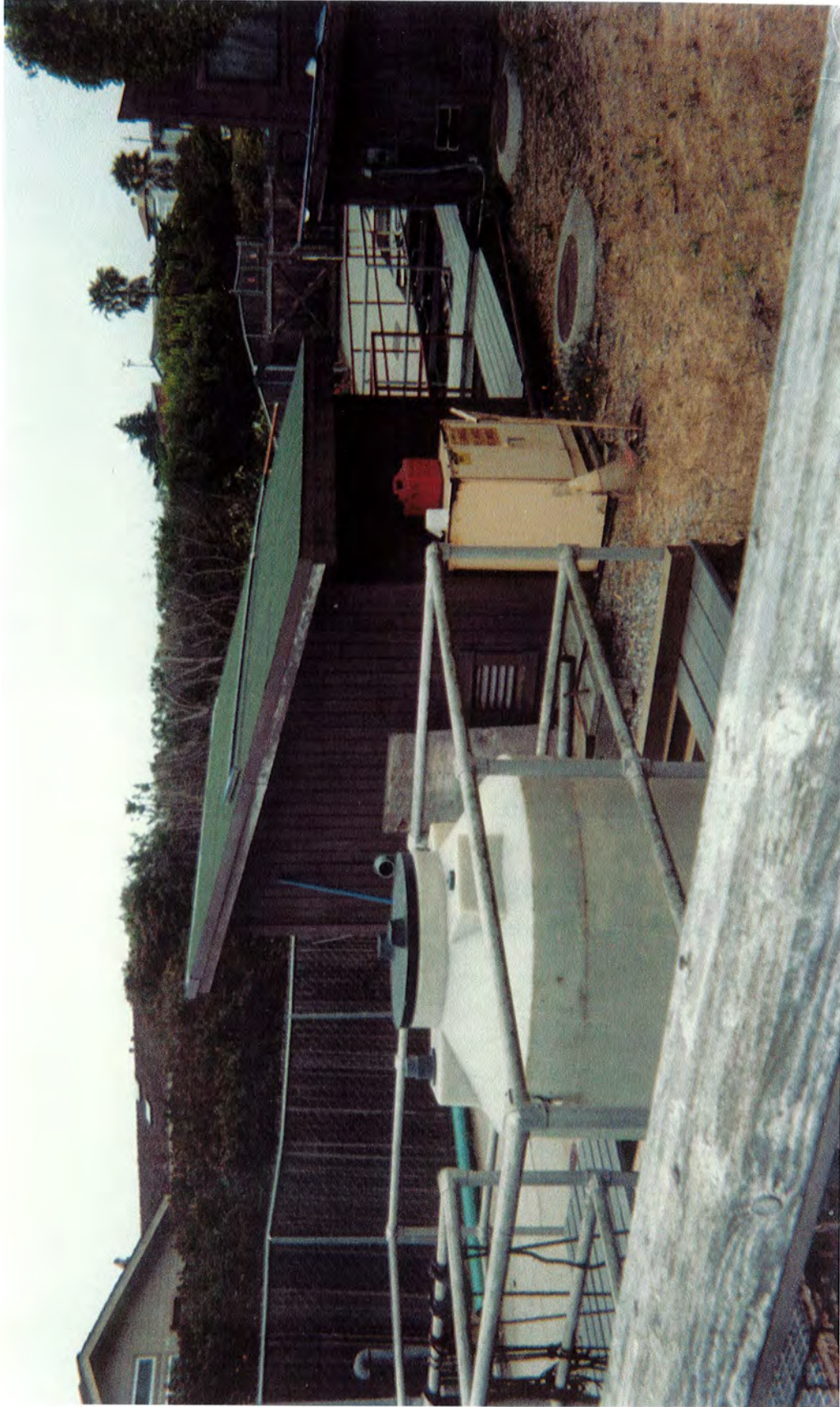
Canon Del Sol - Sewage Treatment Plant Exhibit 5
