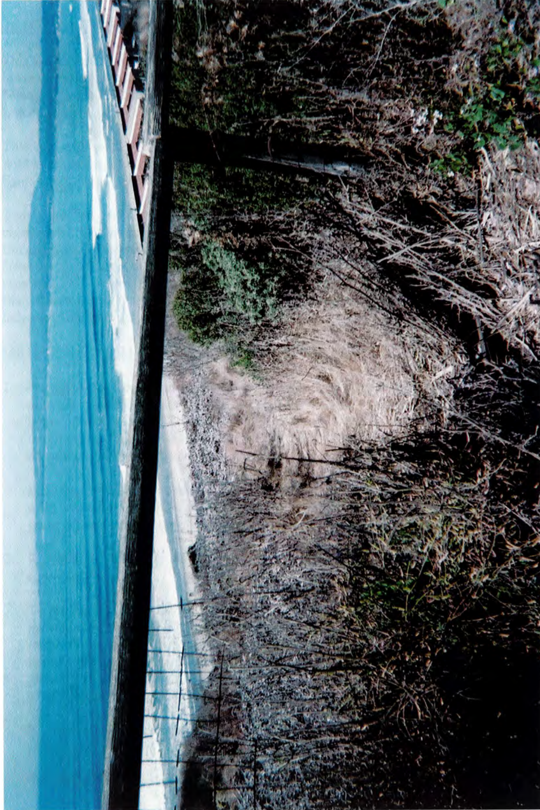
Fence Disrepair Exhibit 9
